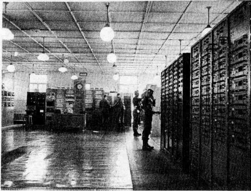
Receiver Operations Room, Camp Owada DCS Receiver Site.
