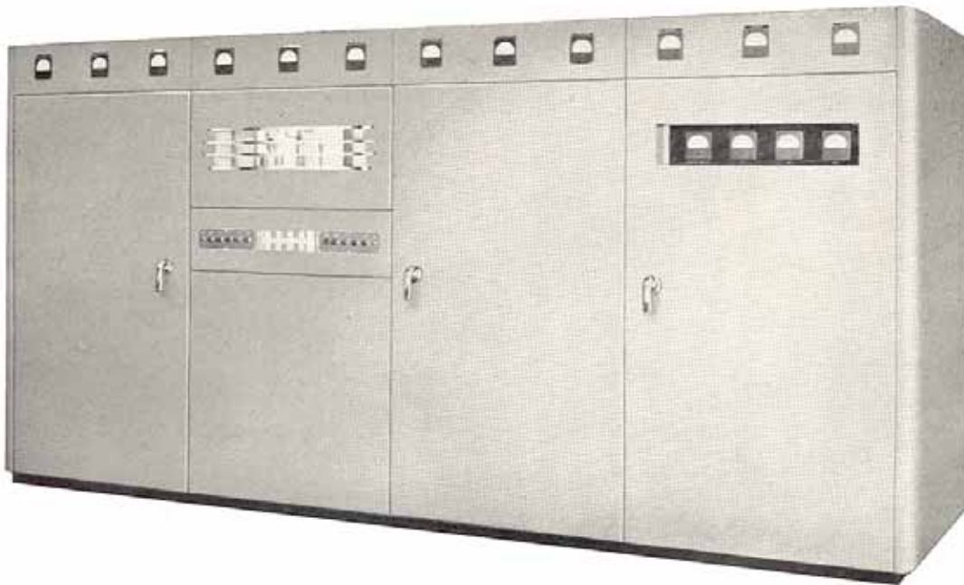
The Transmitter With Phasor
