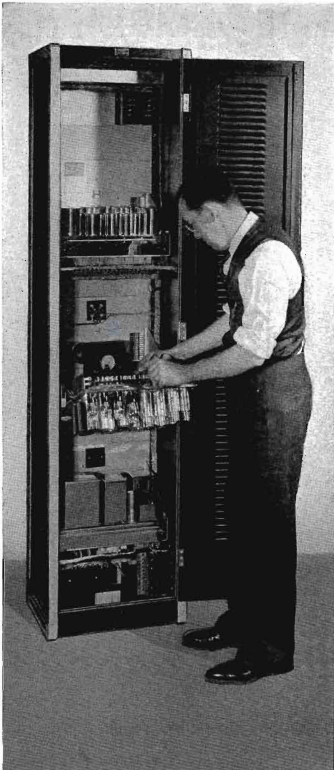
Rear View of 78-B Rack Showing Perfect Accessibility
