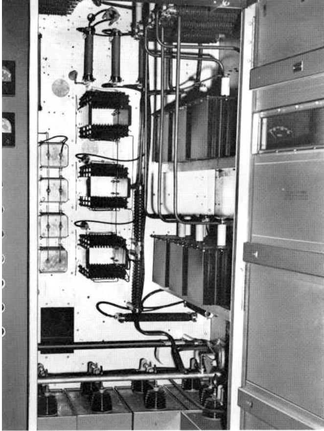
FIG. 4. The new silicon rectifiers are mounted vertically inside the cubicle. Filter capacitors are at the bottom of the cabinet.
