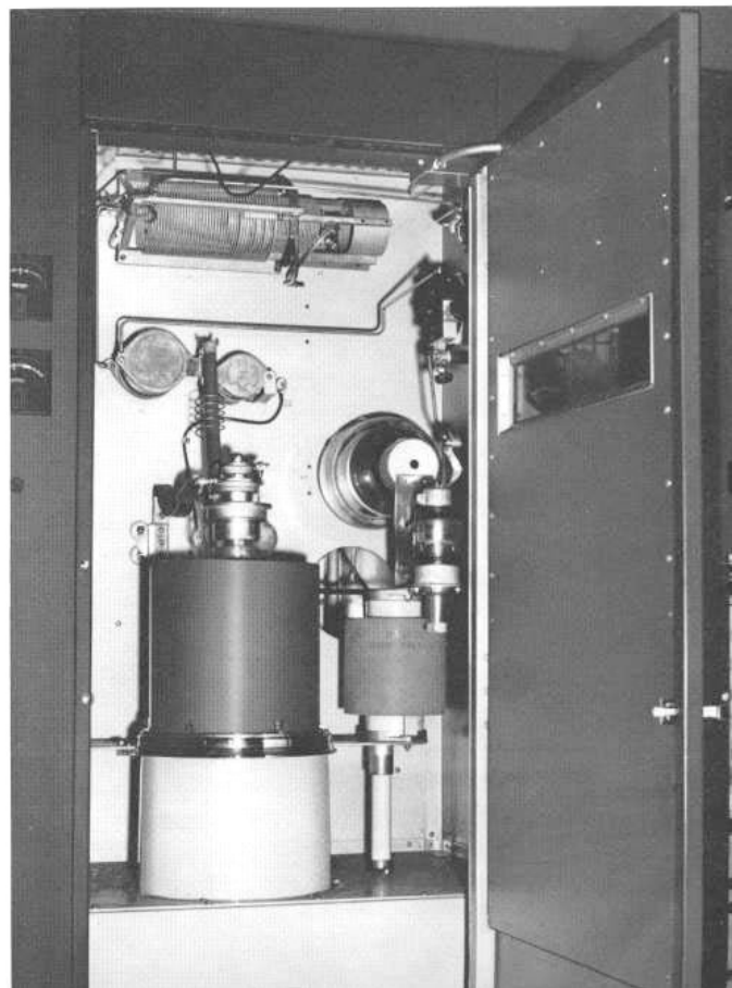
FIG. 3. Close-up of the new PA stage. Note the new lightweight 6697 tube.
