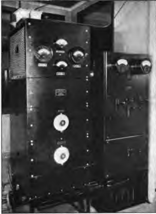
Detroit News Radio Broadcasting Installation. Transmitting panel at left. Control panel at right
