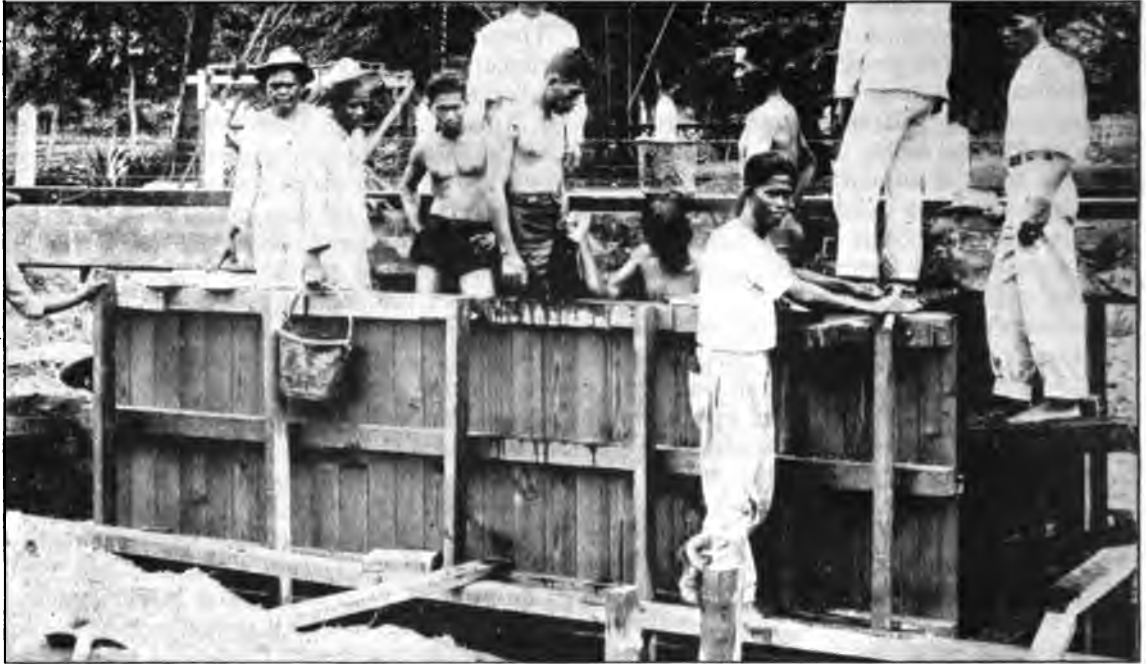
Native Filipinos working on the construction of the Navy's high power radio station at Cavite, Philippine Islands
