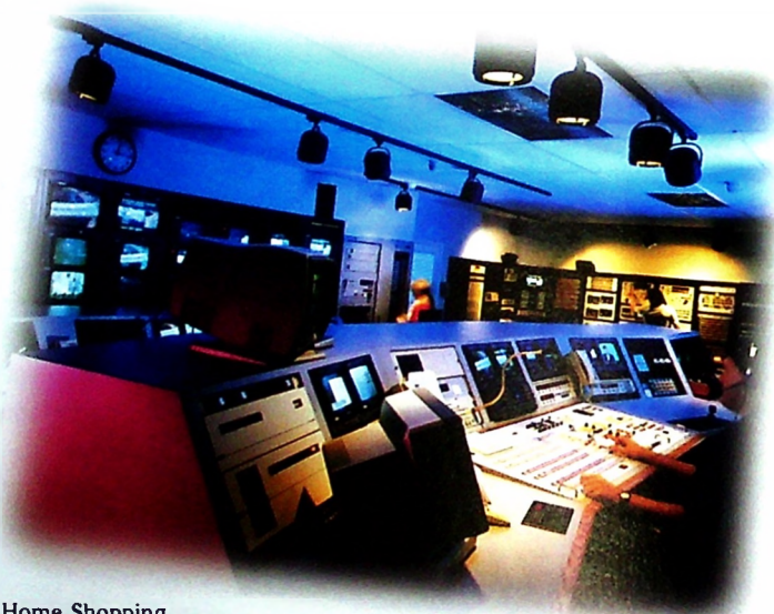
A Home Shopping Network control room, Tampa, Florida
