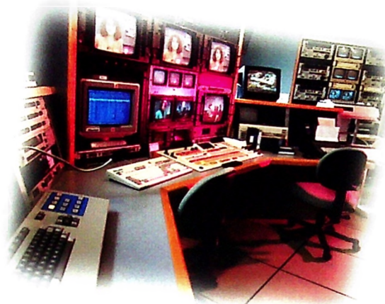
Master Control facility, Disney/MGM Studios, Lake Buena Vista, Florida
