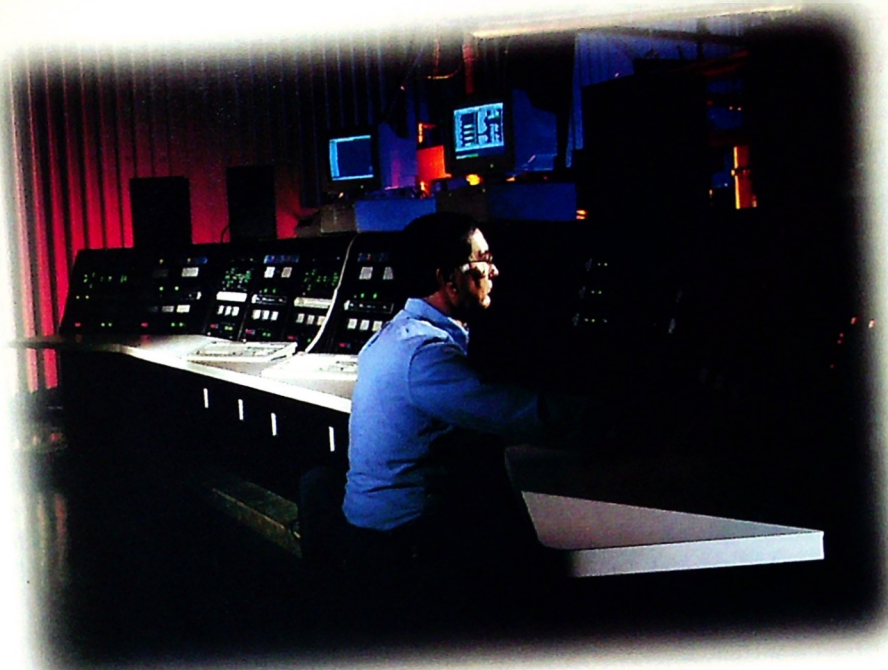
Control console for 120 kW FM system
